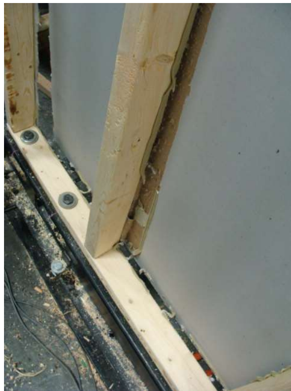
Photo 8: Typical Failure- Bottom Plate
