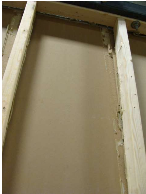
Photo 7: Typical Failure- Top Plate
