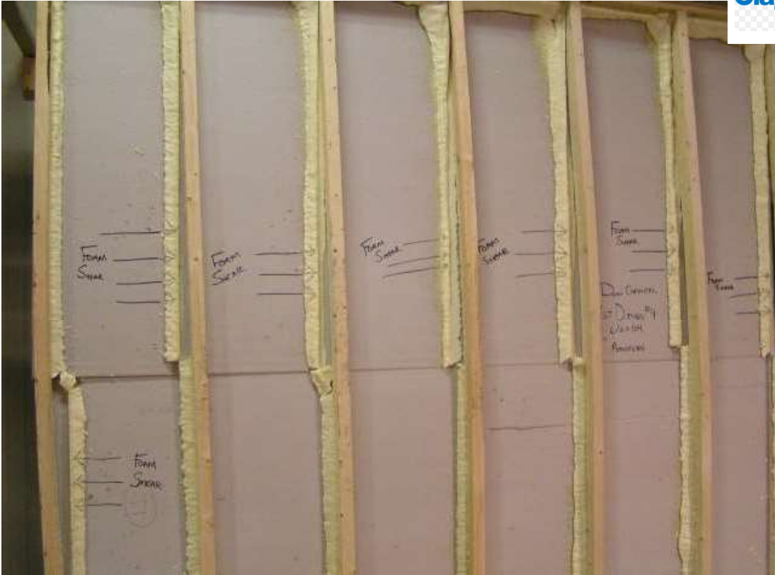
Test #1 stud failure
