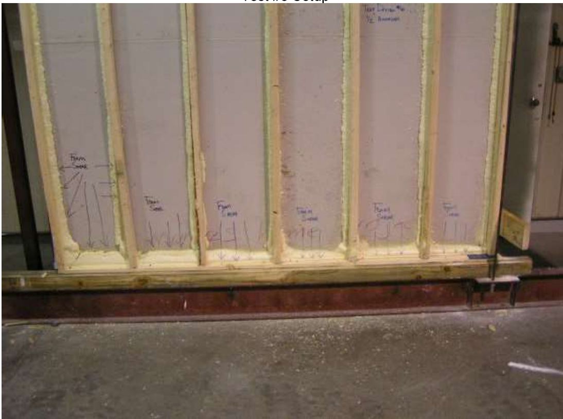
Test #3 bottom plate failure
